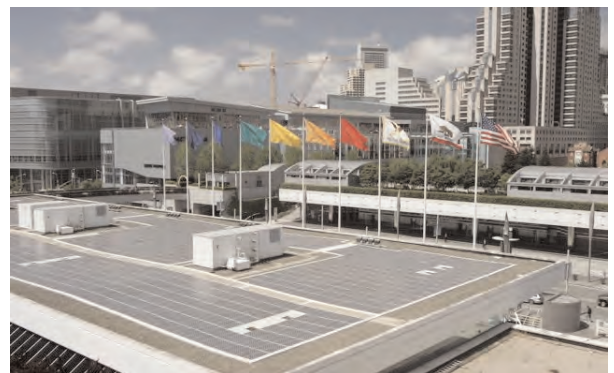
Shell PV modules atop Moscone South's lobby rooftop
